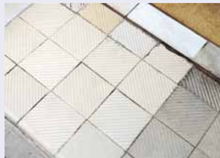
polluted safety tiles
