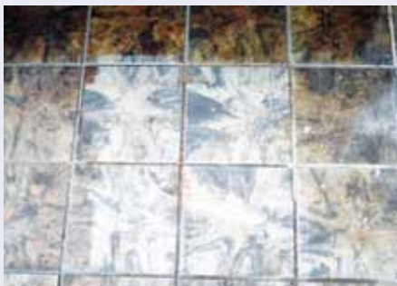
rust on tiles
